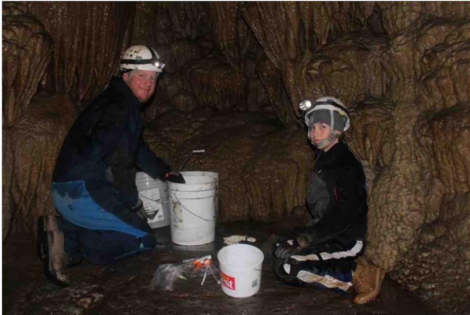
Above: Dean and Parker clean the Paradise Lost pools In Oregon Caves National Monument (OCNM). Bottom right: Swade mixes cement for rimstone repair work: “In case you can’t tell, I’m smiling.” Photos courtesy of OCNM.
